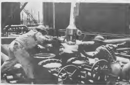
PIPE CRAFT men install the hot tap machine, top photo, on the valve. As W. Bailey, left in bottom photo, watches the indicator, T. Geerman, right, feeds air to the cutter motor.
